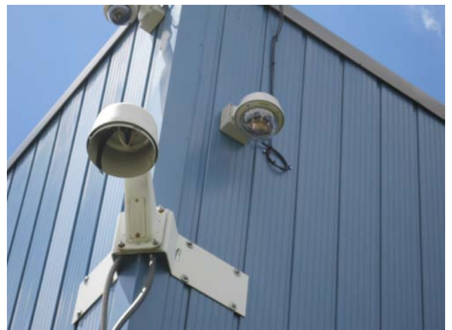
Haynes International installed new IP cameras around the perimeter of the facility to monitor activity.
