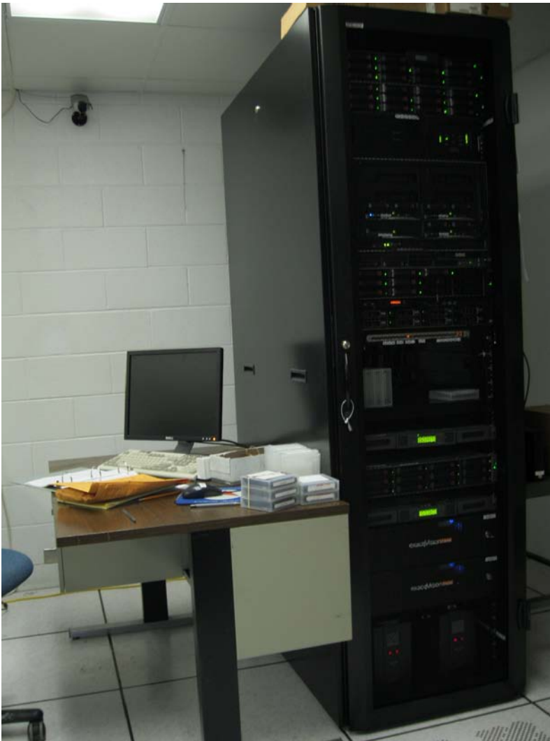
The exacqVision Z-Series servers are installed in the security office.
